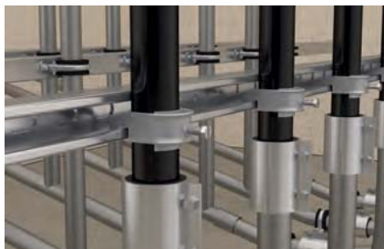
Supply lines fixed to FUS channel
