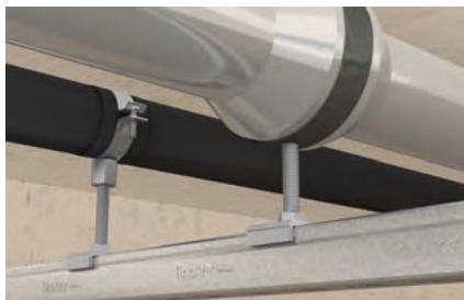
Refrigerant pipe clamps
