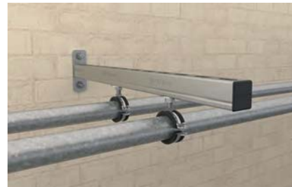
Pipelines on cantilevers
