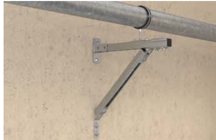
Upright pipe on cantilever arm
